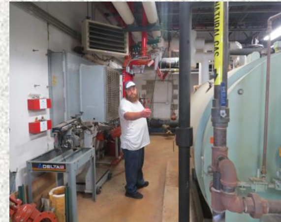
Touring the Boilers
